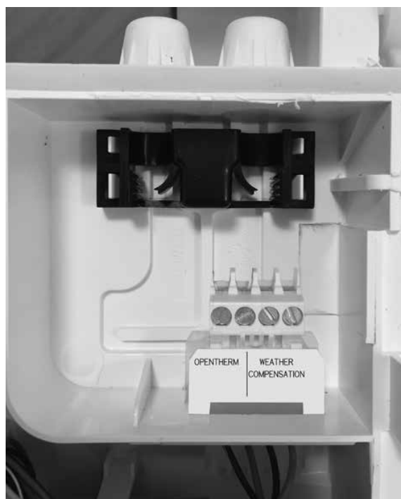
INSTALLER CONNECTIONS (RHS)
