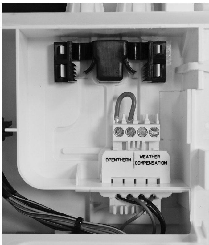
INSTALLER CONNECTIONS (RHS)
