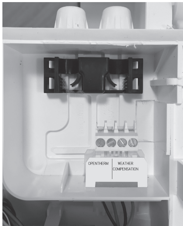
INSTALLER CONNECTIONS (RHS)
