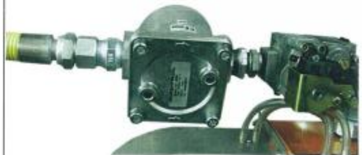
Fig. 32: Mounted gas filter-group at tube heater
