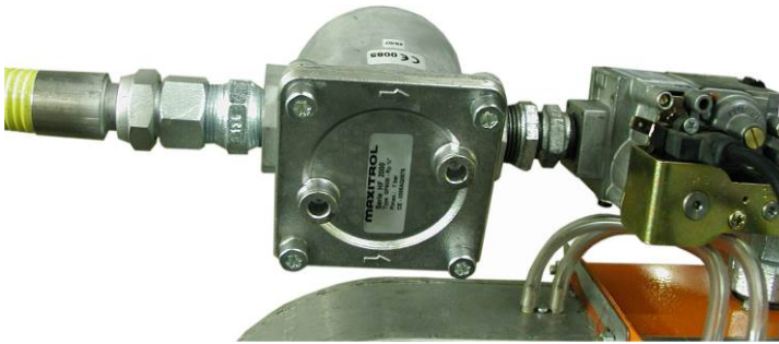
Fig 46: Mounted gas filter-group at tube heater
