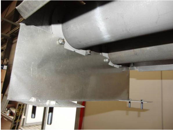
Fig. 35: Fixed end bracket on turnaround box
