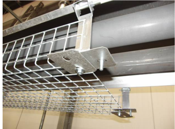
Fig. 38: Loose mounted clamp
